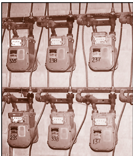
FIGURE 6. Typical meter bank for multifamily building.
